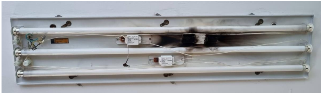
Fig. 7. The extent of damage due to a short circuit of one of the ballasts
