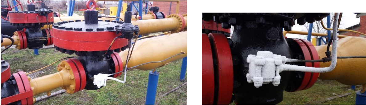
Fig 5. Freezing of gas installation
