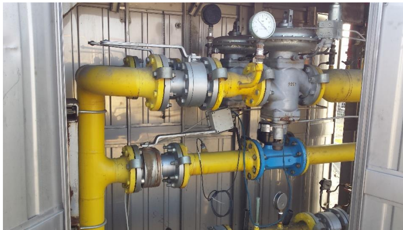
Fig 3. Detail of the installation of the control valve
