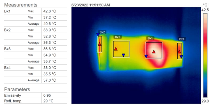
Fig. 3. Thermal pattern immediately after ballast failure
