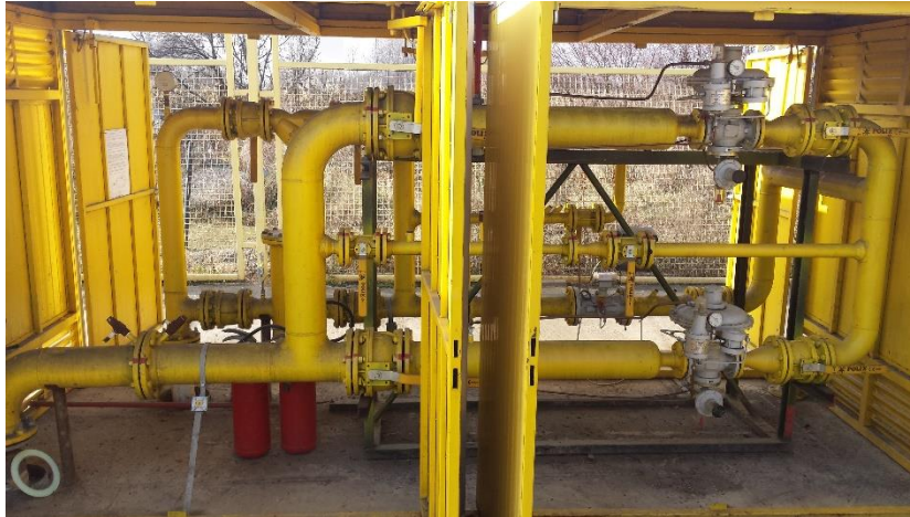
Fig 2. Measuring and regulating station (MRS), with two lines for pressure reduction and a line for measuring gas quantities
